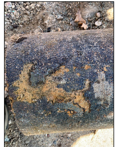
Ductile iron watermain in project area corroded down to concrete pipe liner
