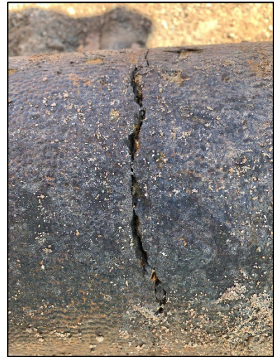
The crack found in watermain that resulted in emergency water shut-off
